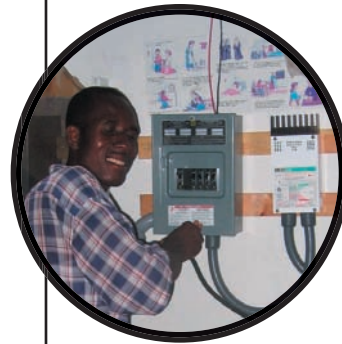
The installation of charge controller and circuit breaker box in a PV system
