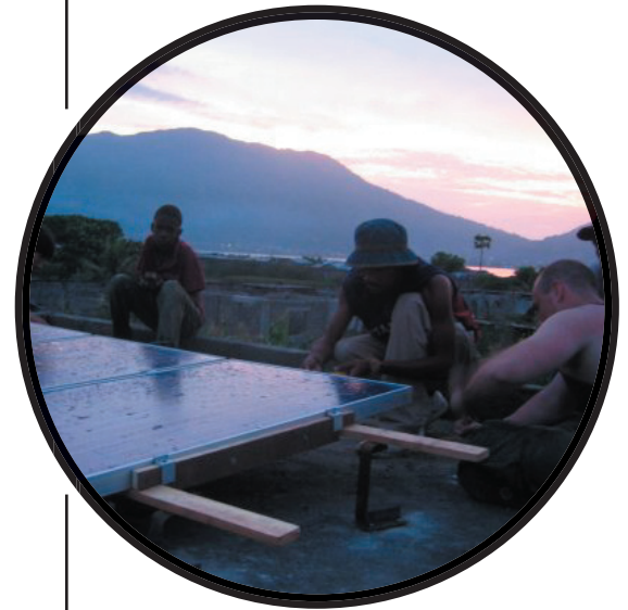
Installing a PV system in a community center in Petite Anse, Haiti
