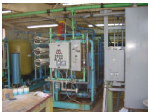
FIGURE 7 CANEEL BAY RESORT DESALINATION PLANT
